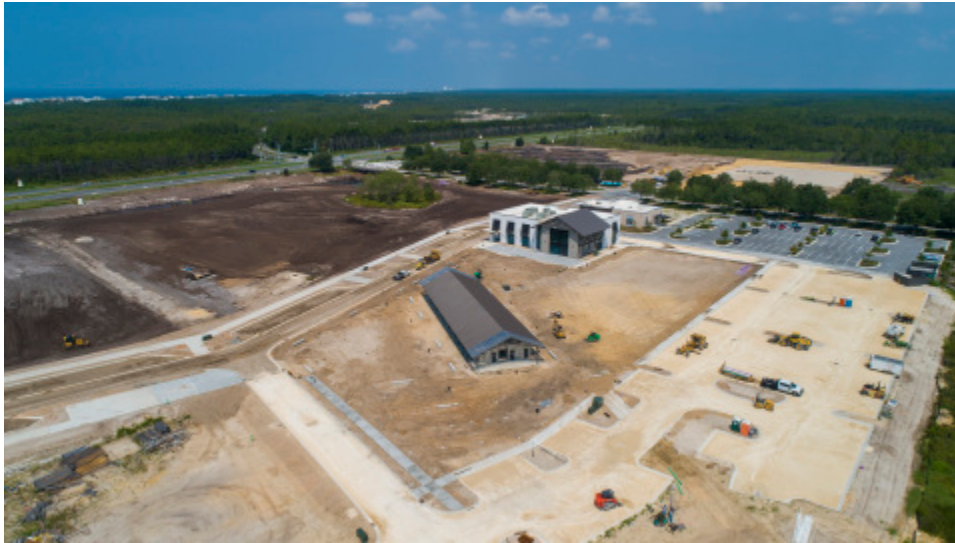
Construction and site work progressing at Watersound Town Center. (Photo: Business Wire)
